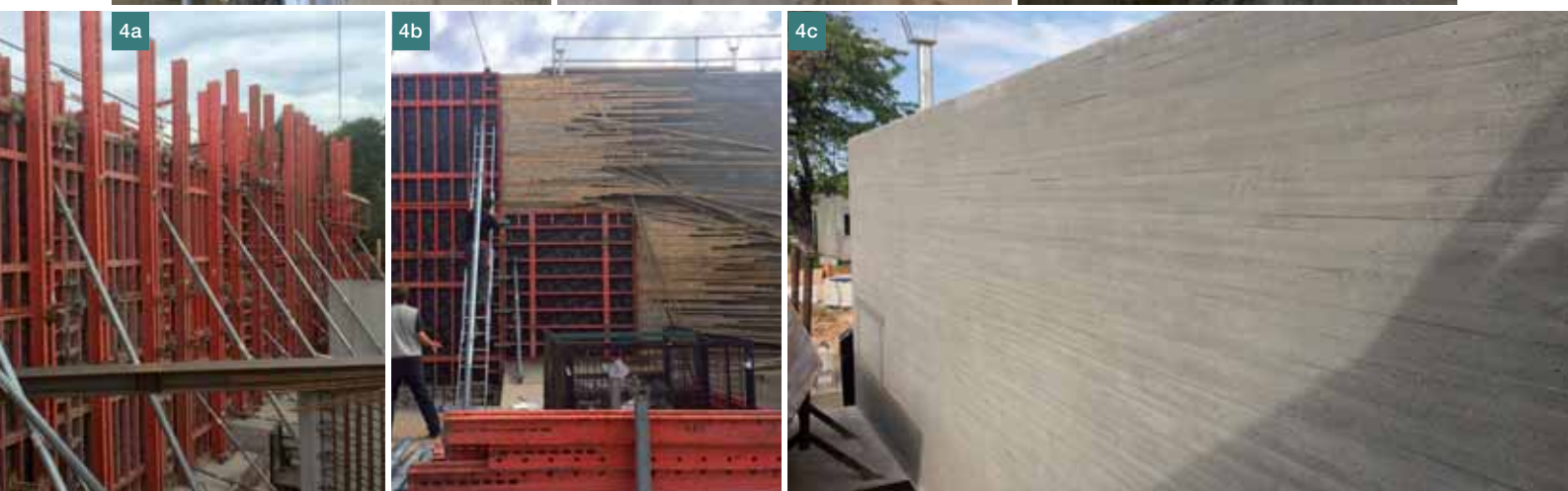
Fig. 3 a) Using the light DUO system for complicated wall concreting under existing slabs, b) hardened cement grout on the surface of earlier concreted bottom part of the wall, caused by insufficiently sealed construction joint during concreting the upper part of the wall, c) not anchored and insufficiently supported formwork broke and moved during strengthening the current structure, it was followed by partial demolition of the structure, d) difficult concreting through small holes in the current structure caused visible stratification, e) incorrectly anchored formwork moved from the bearing wall
